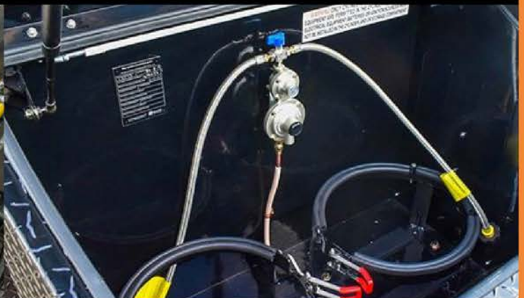
Completely plumbed from gas bottles to kitchen with dual bottle change over valve and gas certification certificate. Additional bayonet gas connection at rear of camper for a BBQ gas supply.
