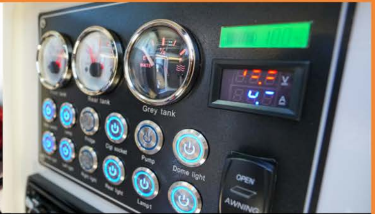
Control panel with water gauges, multimedia system.
